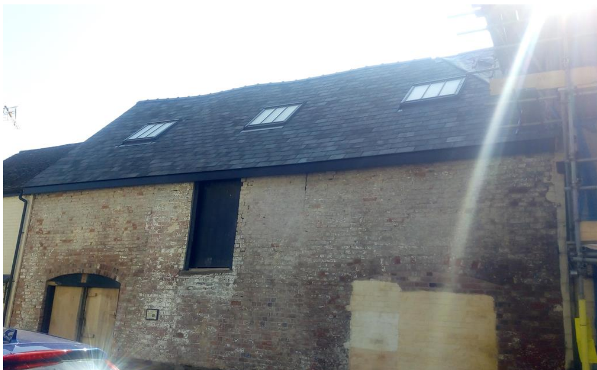
Figure 3: Roof lights in situ when viewed from northern side of High Street
