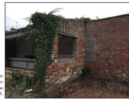
Image 7: Eastern elevation which clearly shows the difference in brickwork between the Glass House and boundary wall.
